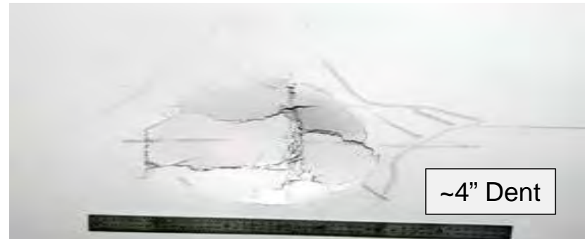
Exterior Skin Damage
